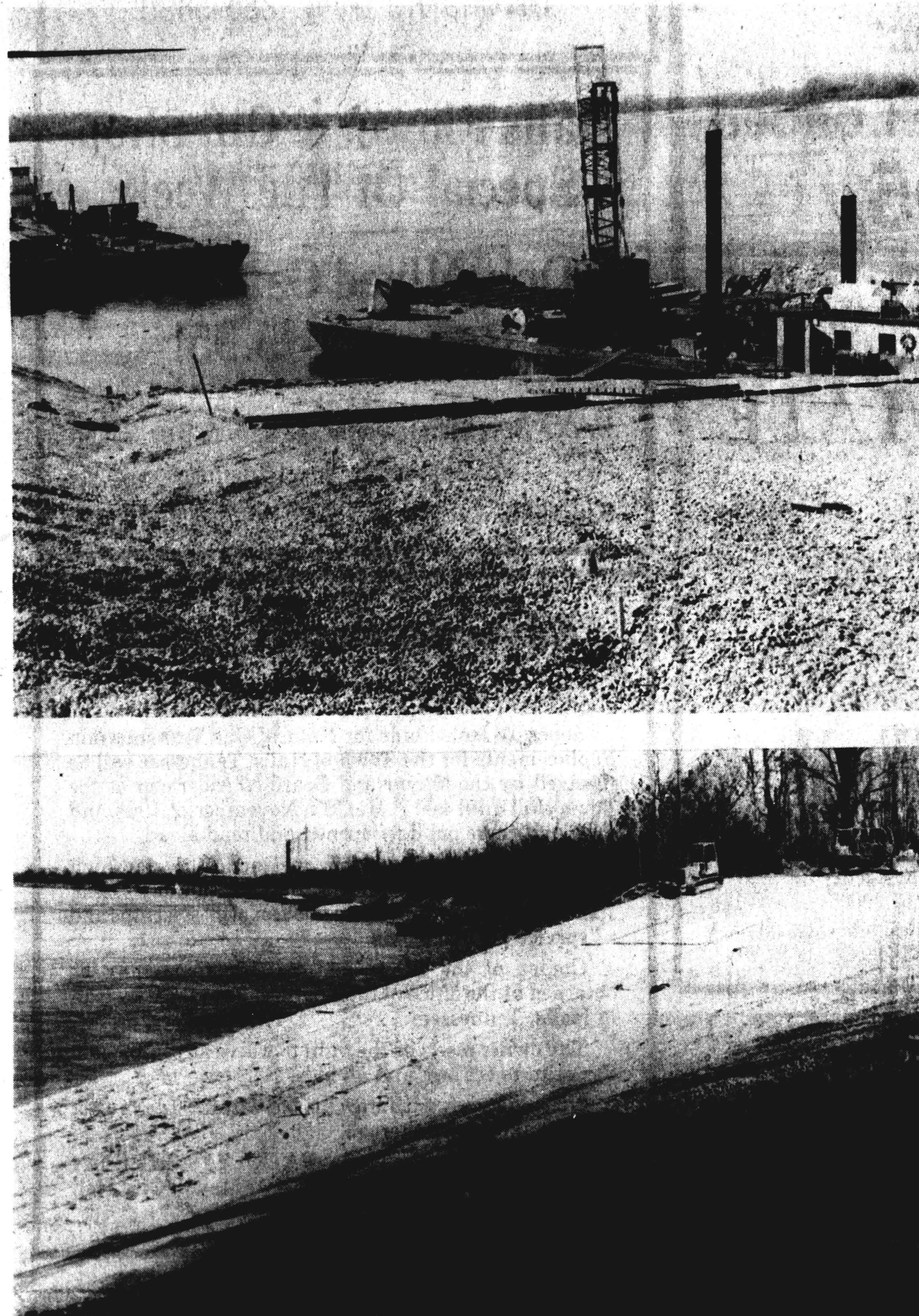
$500,000 BOAT RAMP is near completion at Hale's Point at the Mississippi River.
